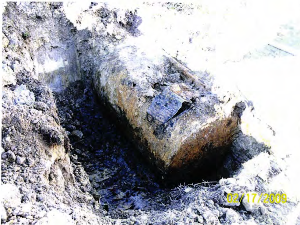
Picture 2: UST 115 Banyan-2 prior to removal from excavation. Tank had previously been filled with sand by others.
